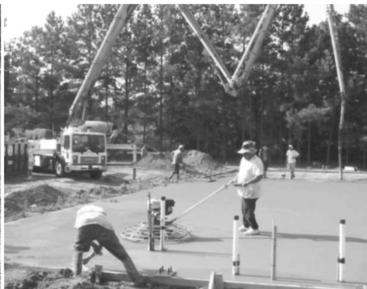
The concrete footings and floor for the new building were poured on July 28th. Shown in background is a boom truck which pumped concrete overhead 65 feet to fill the corners of the site.
