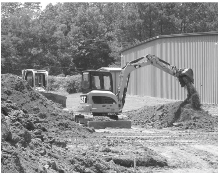
Once site preparation got underway in early July, good weather allowed the construction to move at a good clip on the new Sporting Dog Wing at the National Bird Dog Museum.
