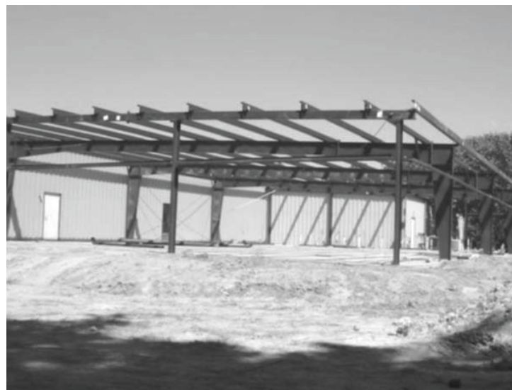
The new Sporting Dog Wing at the BDF will create nearly 6,000 sq. ft. of added exhibit space. The steel for the structure was erected most recently and now has a roof and walls added.
